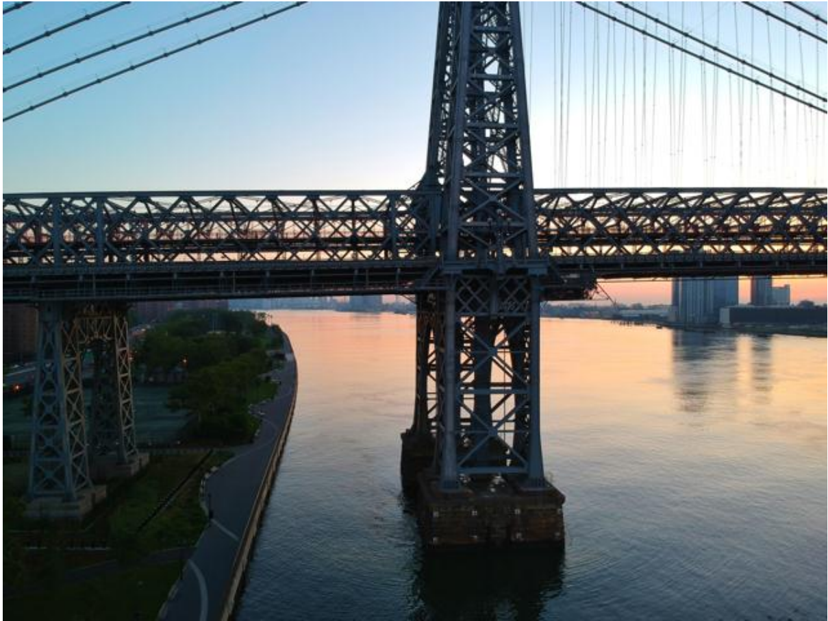
Bridges across the country require constant repainting. Image credit: Unsplash User Jeffrey Blum
